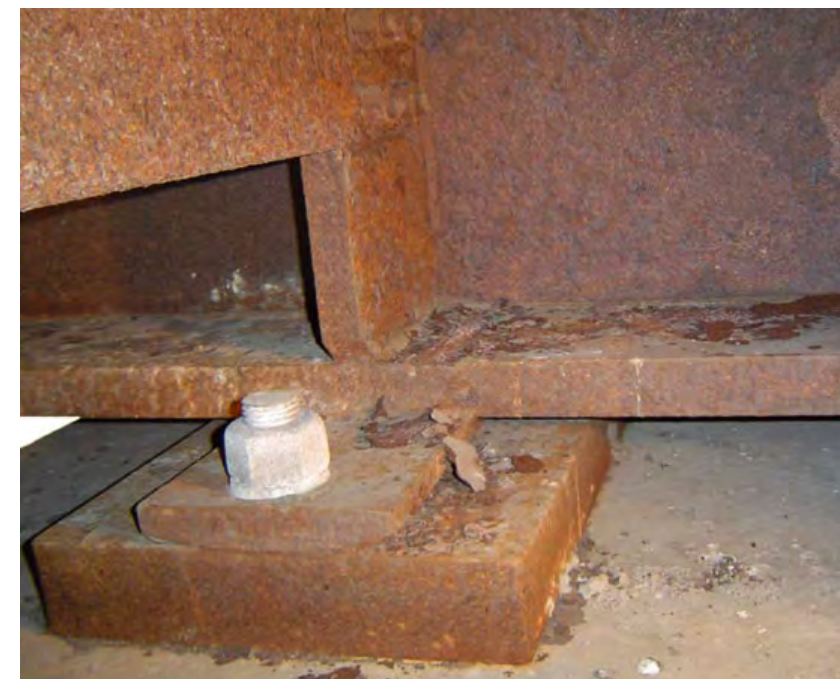
Excessive corrosion on weathering steel beam and bearing plate.
