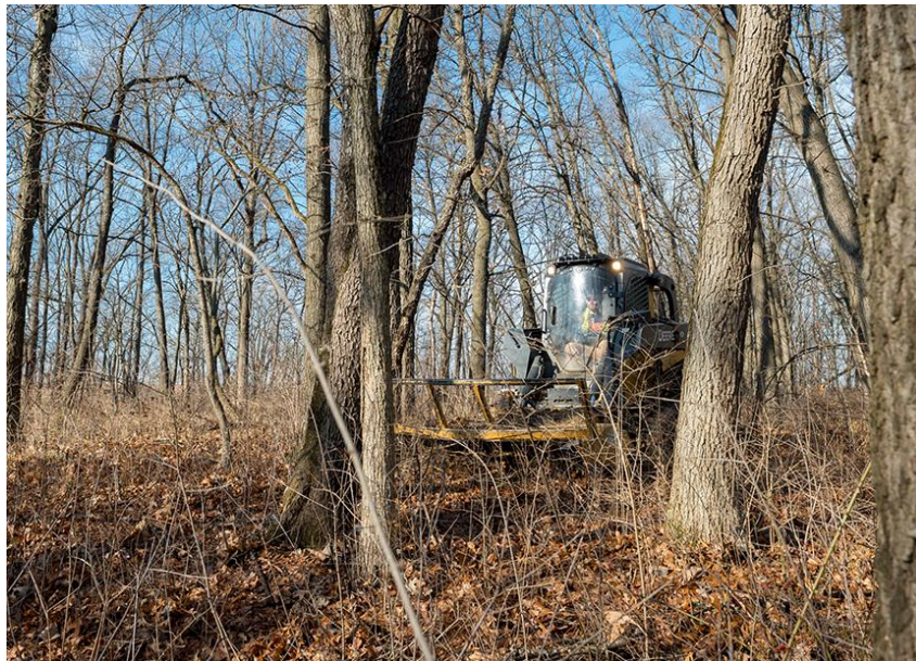
Figure 10. Argonne Infrastructure Services grounds staff member operating a skid steer forestry device. Photo: Argonne National Laboratory
